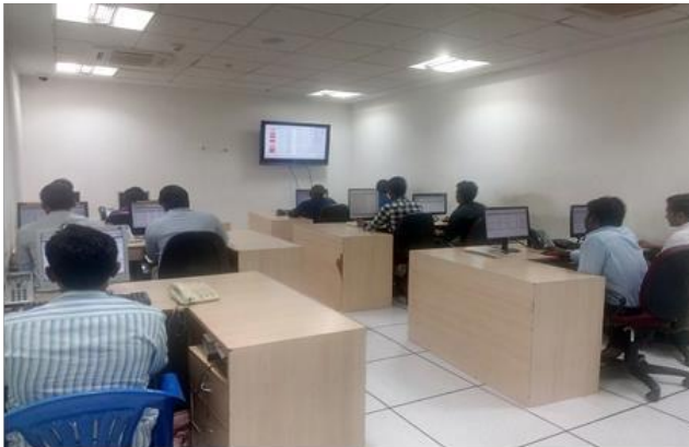
Network Operation Centre of TNSWAN
