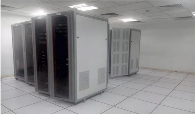
Network Room of TNSWAN (Figure-19)
